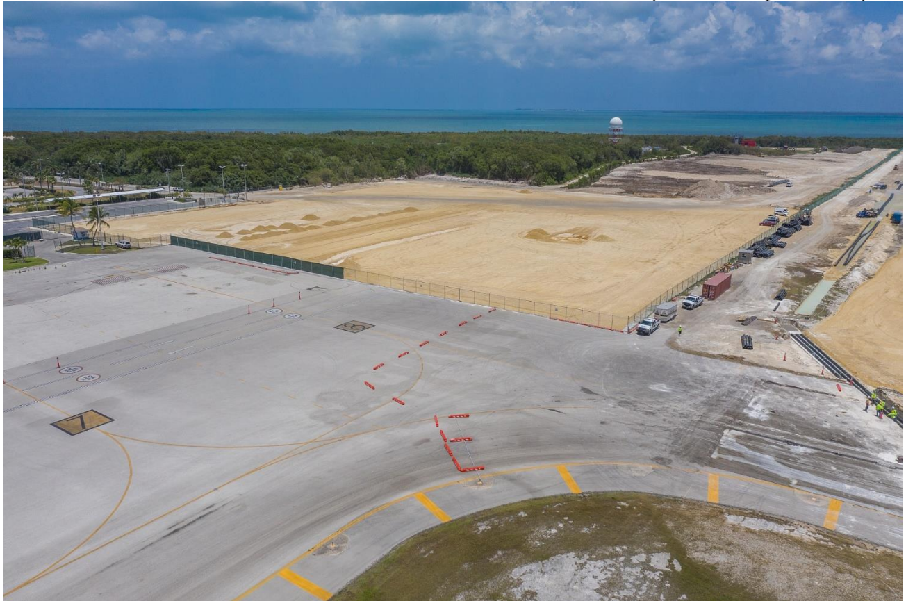
PHOTO 2 SUBMITTED: Easterly view of the new Apron Expansion at Owen Roberts International Airport, which will have the capacity of parking four aircraft
